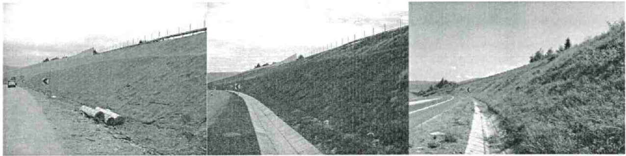
Figure 3: Example of a pinned mesh slope (during installation, immediately after revegetation, and with developed mature grass).
